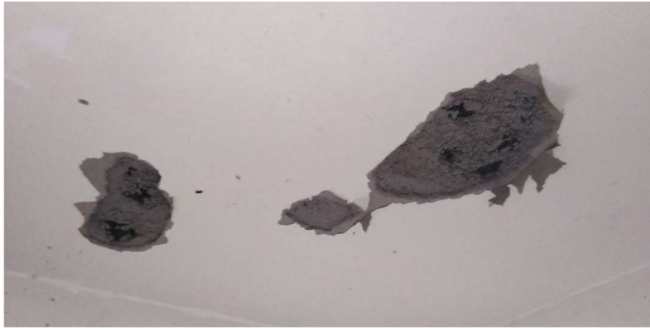
Section of the ceiling in the guardhouse that need repairs
