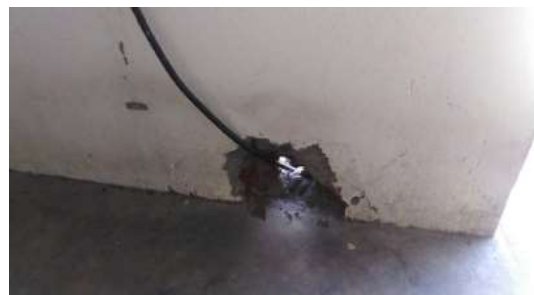
Cable from the borehole to the pump house, repairs need to be done
