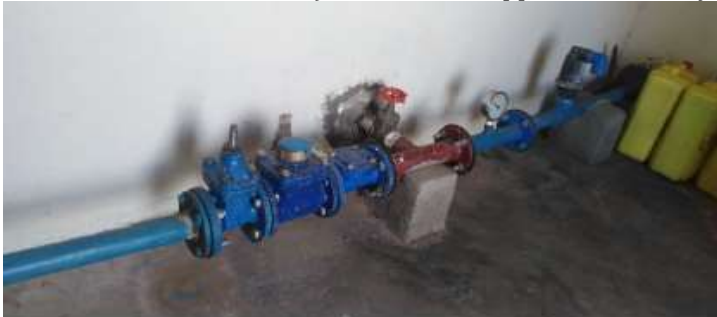
Well head fittings
