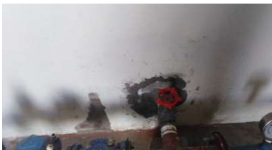
Area that need repairs
